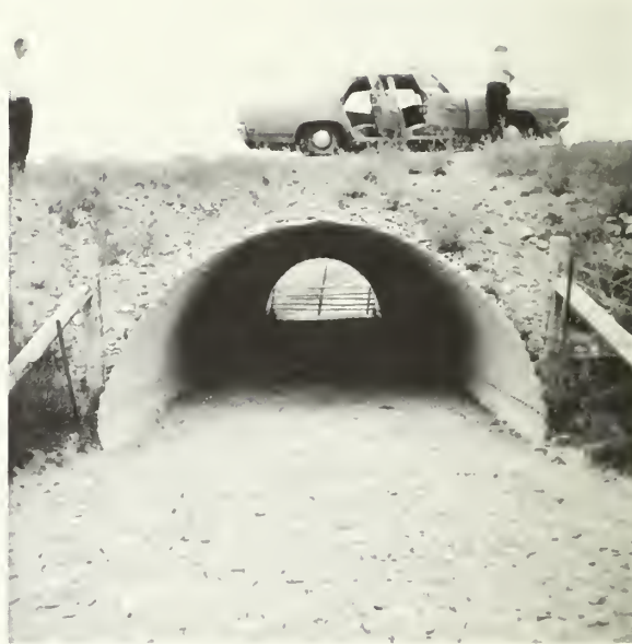
WEST ENTRANCE; water collects and area becomes a quagmire of mud. Very poor drainage.
